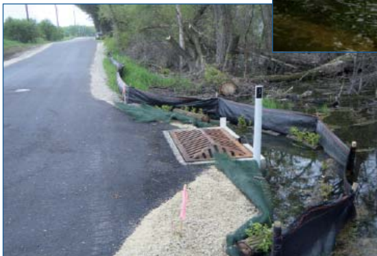
Water from lowlands enters outlet structure at Lower Lake Road
