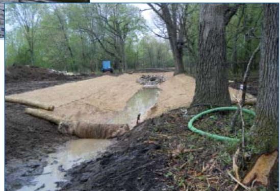
Water leaves outlet pipe through discharge point and swale (shown under construction)
